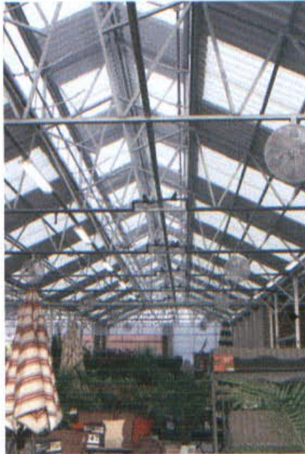
Clerestory panels reduce store lighting needs.
